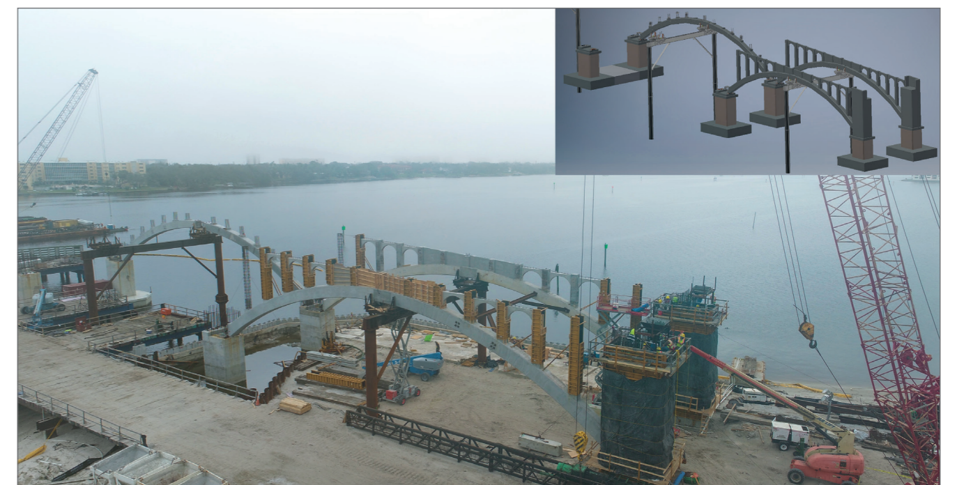
Fig. 11 Approach Span Precast Arch Ribs on Falsework Towers [1] with Integrated 3D Bridge Model Rendering (Top Right)
