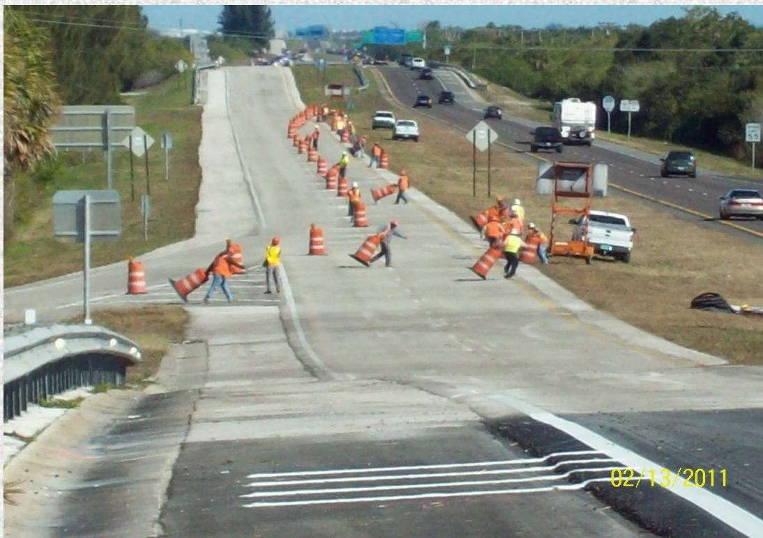
Two days later the barrels were removed to allow the traffic onto the bridges.
