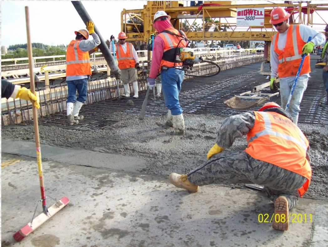
Seven days after the beams were set, the bridge decks were ready for concrete. The contractor used stay in place forms for the bridge decks.
