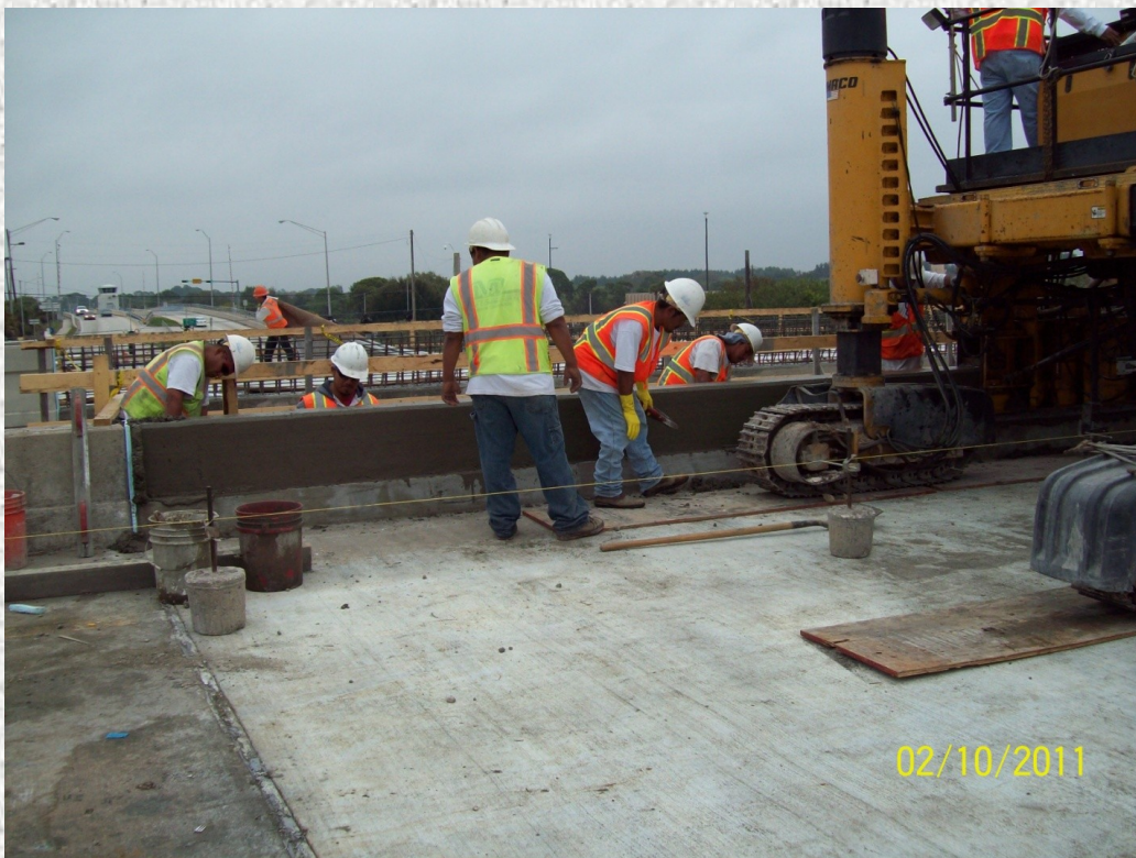
Two days after the decks were poured; the barrier walls were slip-formed.
