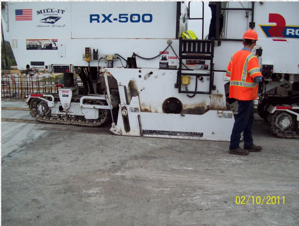
While the barrier walls were being placed, milling of the SR-528 pavement occurred.
