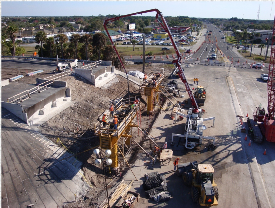
Monolithic concrete pour of the columns and pier caps. This type of pour saved the contractor three (3) days. The forming of the columns and pier caps was accomplished in four (4) days.
