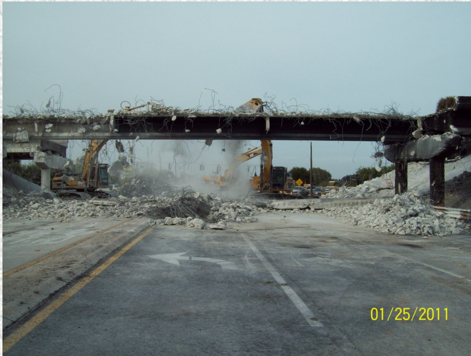
The bridges were demolished in two (2) days by the giant concrete eaters.
