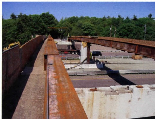
The I-girders of the original steel bridge were removed and then reused as temporary erection beams to support the precast concrete channel segments during erection.
