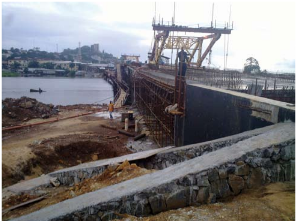
End Span Closure Segment completed using form traveler New Vai Town Bridge, Monrovia, Liberia.
