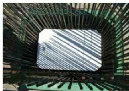
Polystyrene was used in the hollow pier columns, except at the base and caps, which are solid. This eliminated the need for interior formwork and reduced the overall mass of the structure and the amount of concrete required.
