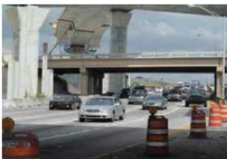
This is a major route to Miami International Airport (MIA), with more than 430,000 motorists using the interchange daily.
