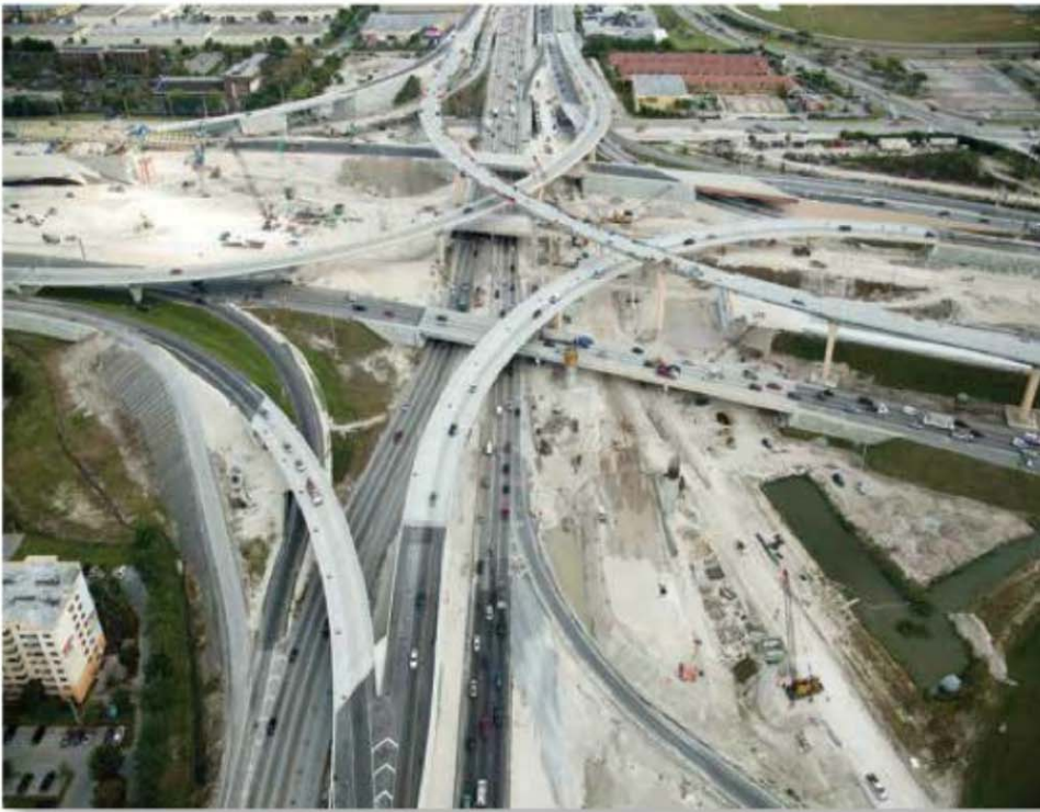
Bridge 9 is under construction as of April, 2014. Photo courtesy of Smith Aerial Photos.
