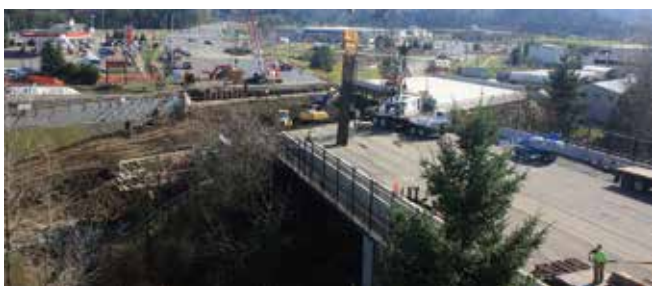
The old bridge has been removed and the new bridge is ready to be moved into place.
