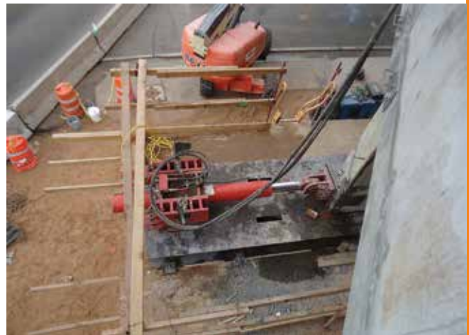
On the West Mesquite Interchange at I-15 in Mesquite, Nev., hydraulic jacks were used to push the bridge into place. All photos: Jackie Borman, HDR.
