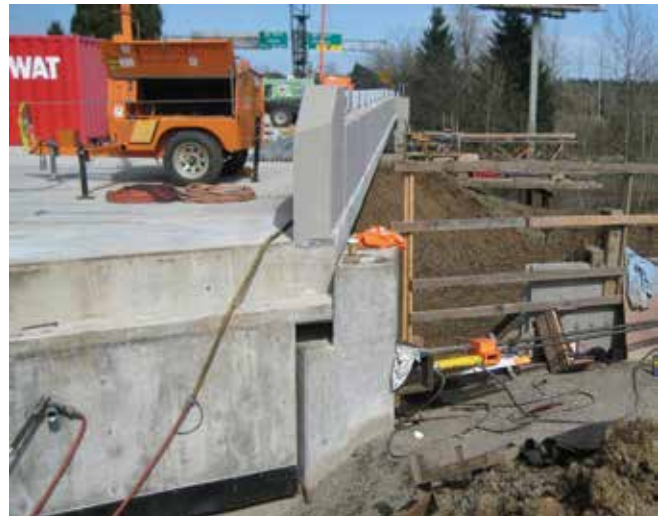
This before and after view shows how the abutment was changed once the bridge was moved into place. Note the channel guide rail and tension rods.
