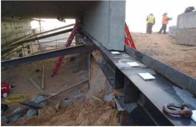
Teflon pads on rails assisted in sliding the approach slab and bridge into place on the West Mesquite Interchange at I-15 in Mesquite, Nev.
