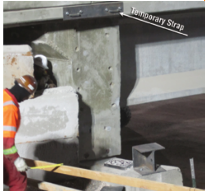
Temporary strap tying the approach slab to the bridge deck slab. Photo: Horrock Engineers.
