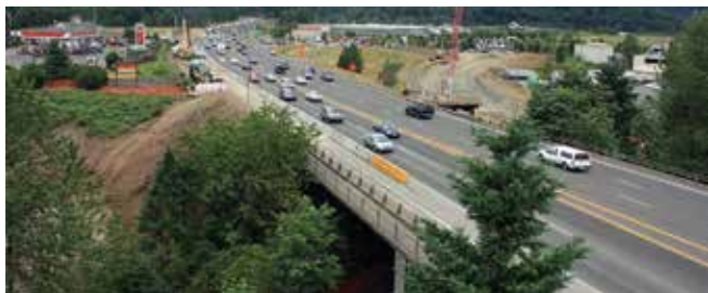
Construction of falsework for the new bridge begins on the right side. All photos: Hilman Rollers.
