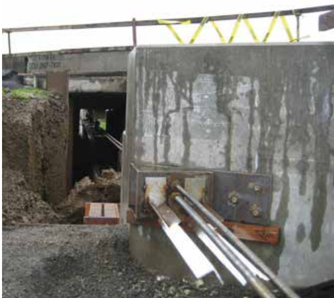
Tension rods are anchored at the abutment to create a reaction point. Note the bracket to accommodate the skew of the bridge.
