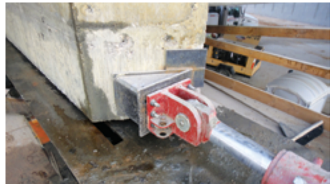
Push block between the hydraulic jack and the abutment must handle an axial load plus a horizontal shear without damaging the end of the diaphragm. Photo: Horrock Engineers.
