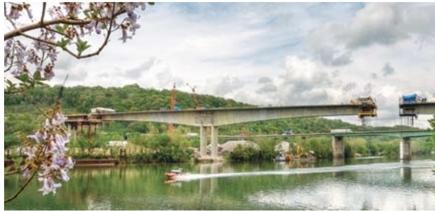
Figure 1 - Kanawha River Bridge main span before closure. (Photo courtesy of T.Y. Lin International).
