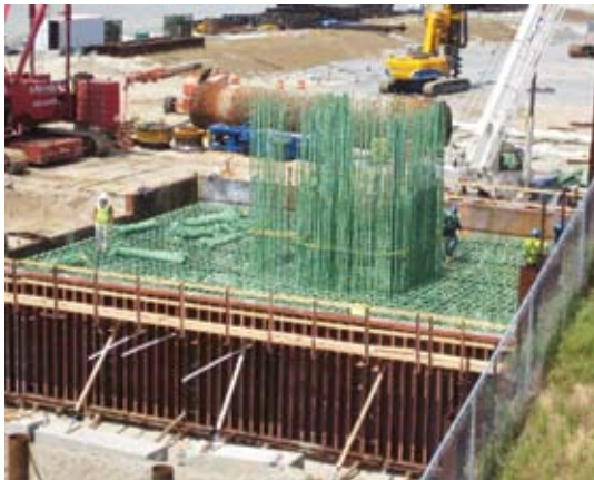
Figure 15 - The current construction progress as of the end of August 2009 includes 80% of the 36" square prestressed concrete pile foundations have been driven to 1800 ton capacity; pylon footing and tower construction has begun (photo of Northeast Pylon footing); and installation of temporary falsework used for the cable stay superstructure erection over land has begun. (Photo courtesy of AECOM).
