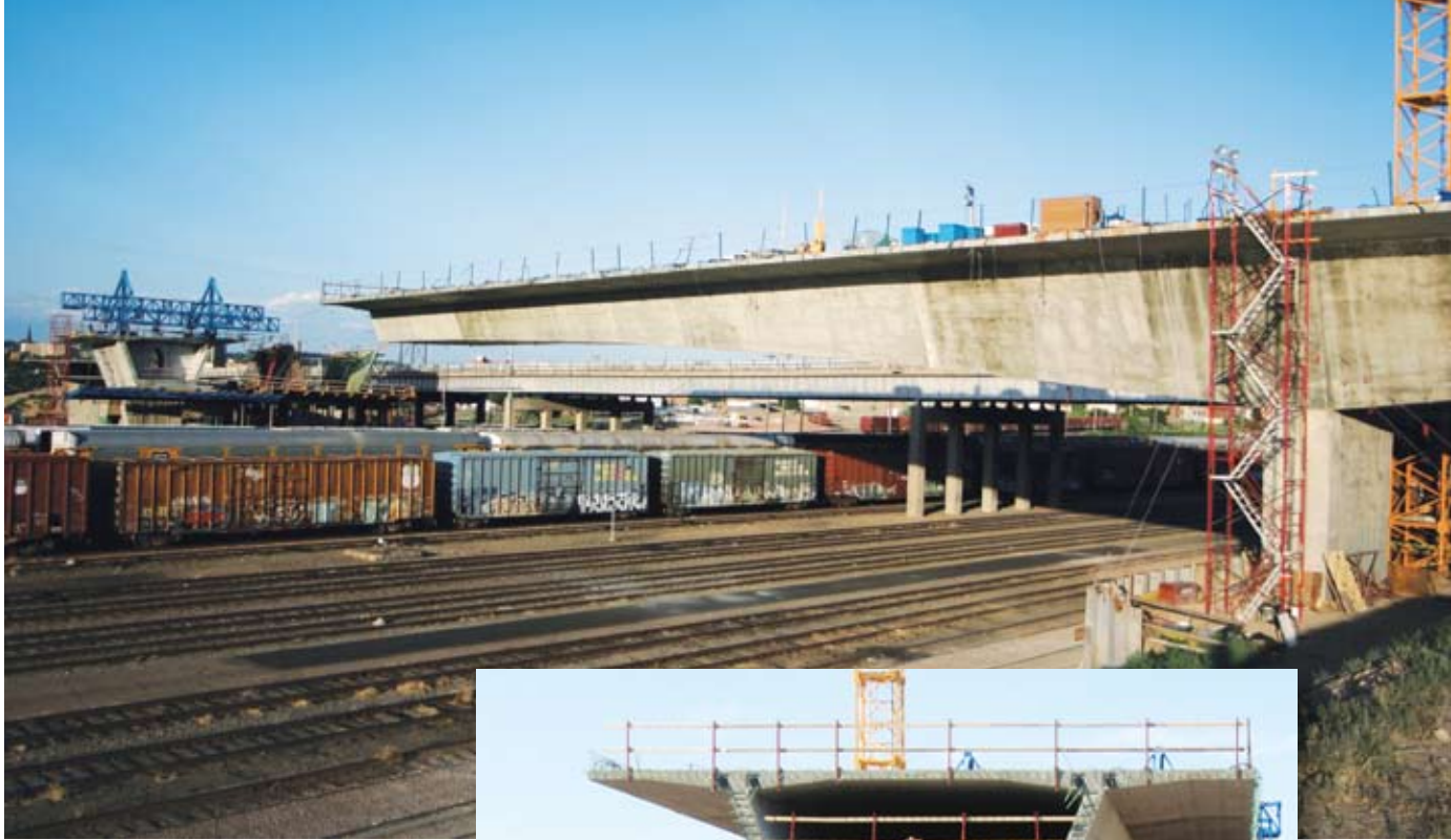
Figure 6 - (Photo top) July 2009 - Variable depth cantilevers extend out 192' to form a gentle arch over the rail yard while maintaining appropriate clearances for construction. (Photo courtesy of FIGG).
