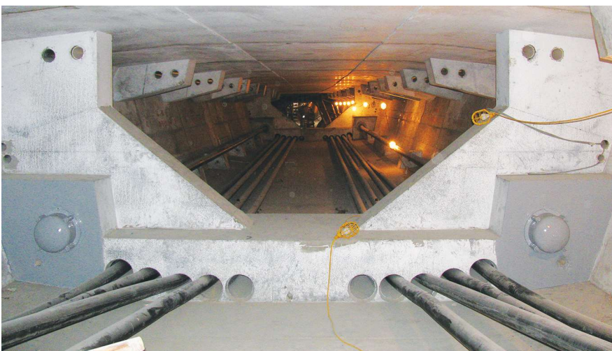
Deviation segment showing the diabolos with external tendons installed. Photo: Florida Department of Transportation.
