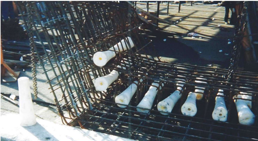
Diabolo void forms placed in a precast concrete segment. Photo: Finley Engineering Group Inc.
