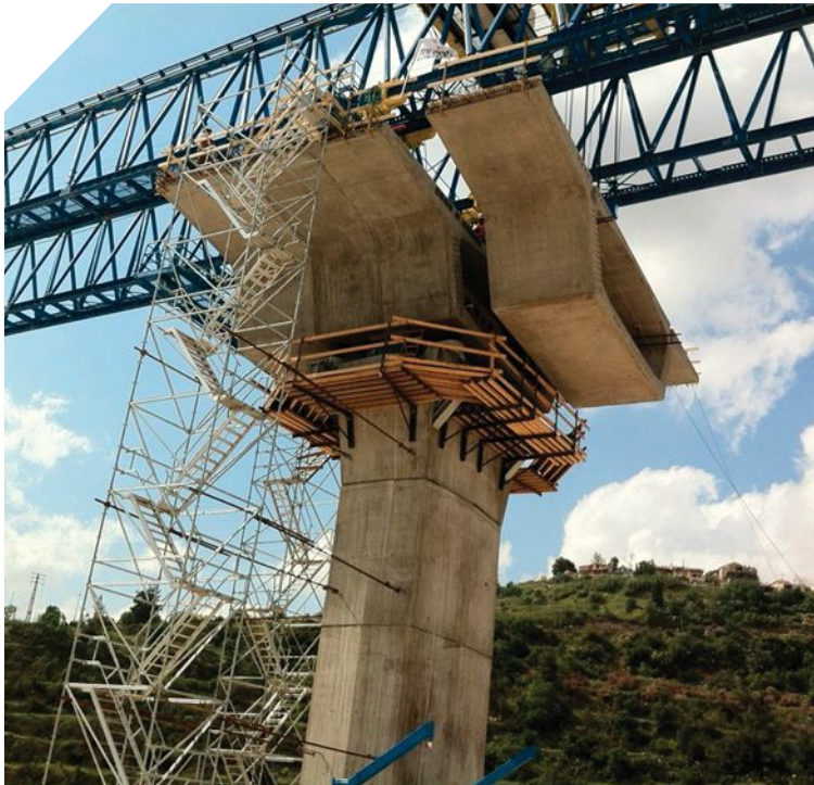
Potucek has recently been working on the Motzha Bridges near Jerusalem, Israel.
